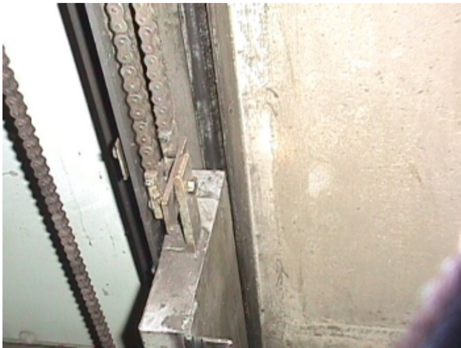
Figure 4. Gate Counterweight Connecting Bolt Assembly
